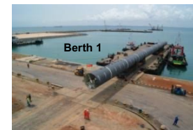
Berth 1 ( length 130 m ) - for Tug & barges up to 2,000 DWT with water draft up to 5m LWS
